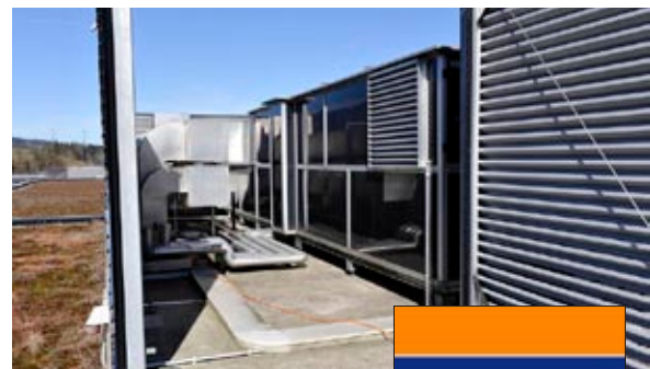
Heat pump system at Nikon AG
