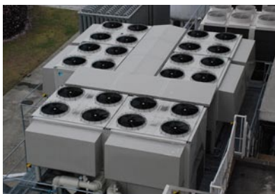
Heat pump chiller equipment of the seamless HVAC system
