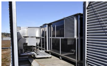
(Right) Heat pump system (Nikon AG) (Left) Certificate for green electricity (Nikon Europe B.V.)
