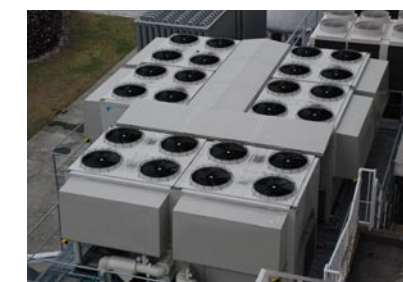
Heat pump chiller equipment of the steamless HVAC system
