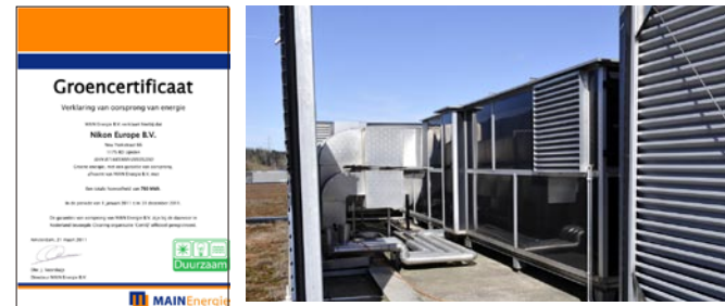
(Right) Heat pump system (Nikon AG) (Left) Certificate for green electricity (Nikon Europe B.V.)
