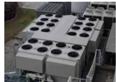
Heat pump chiller equipment of the seamless HVAC system (Tochigi Nikon Precision)
