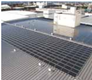
Solar power generation panel (Kumagaya Plant)
