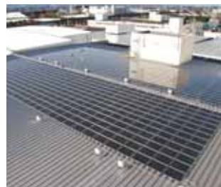
Solar power generation panel (Kumagaya Plant)
