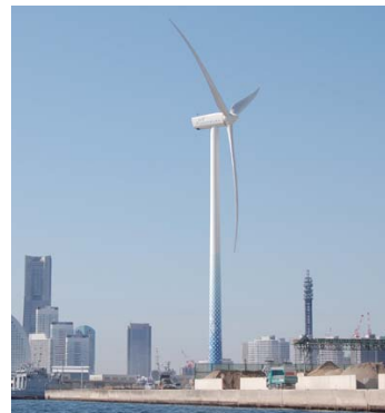
Hama-Wing (Yokohama City wind-power plant)
