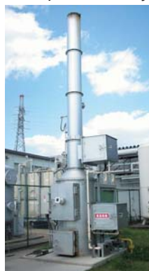
Gasification furnace (Sendai Nikon)
