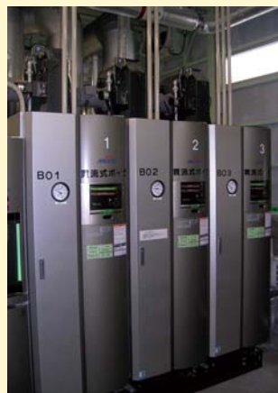
High-efficiency boilers fueled by town gas
