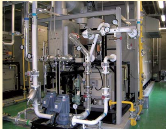
Cogeneration equipment that recovers & uses waste heat to supply electrical power during the daytime
