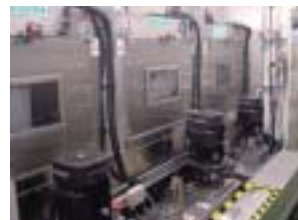
The all-water washing system at Yokohama Plant.
